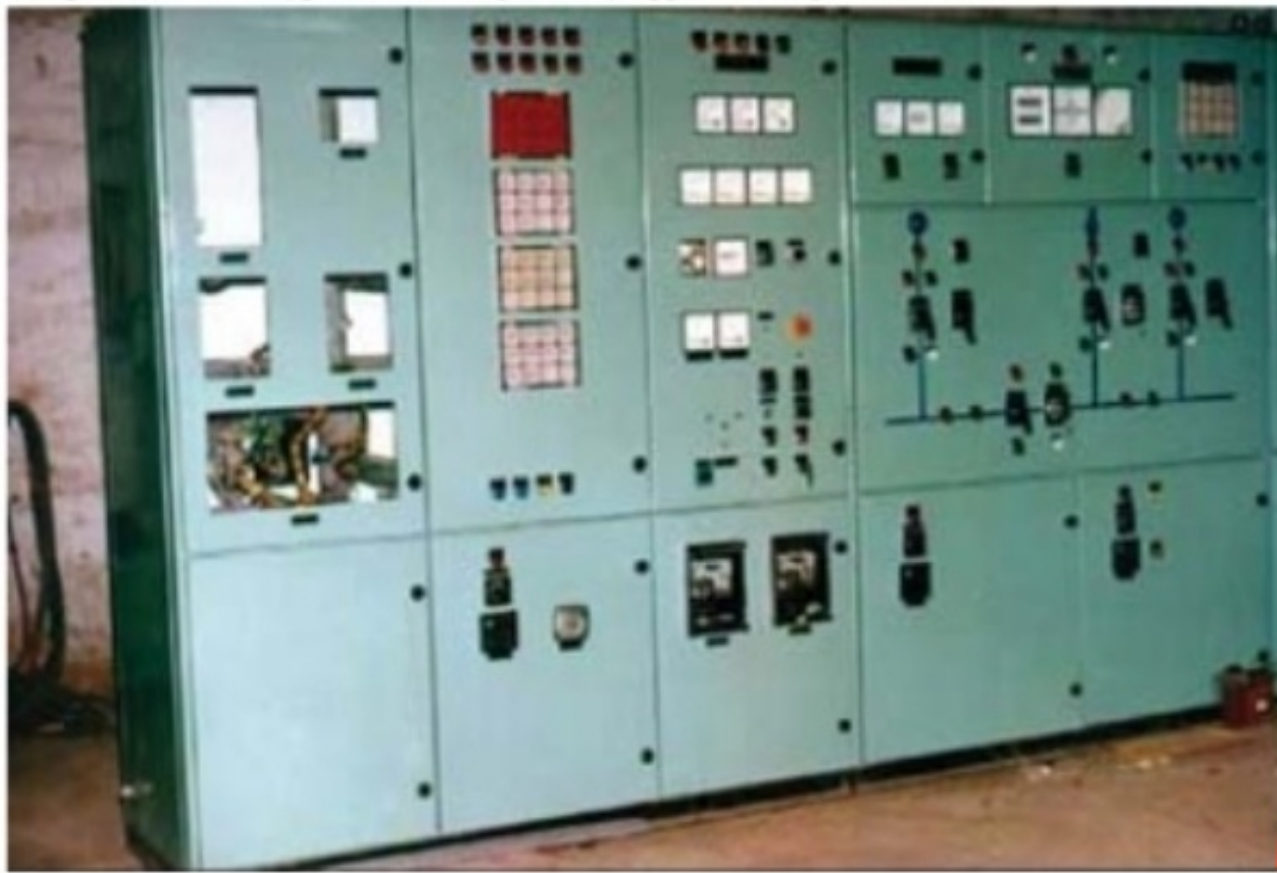
Power Factor Improvement
